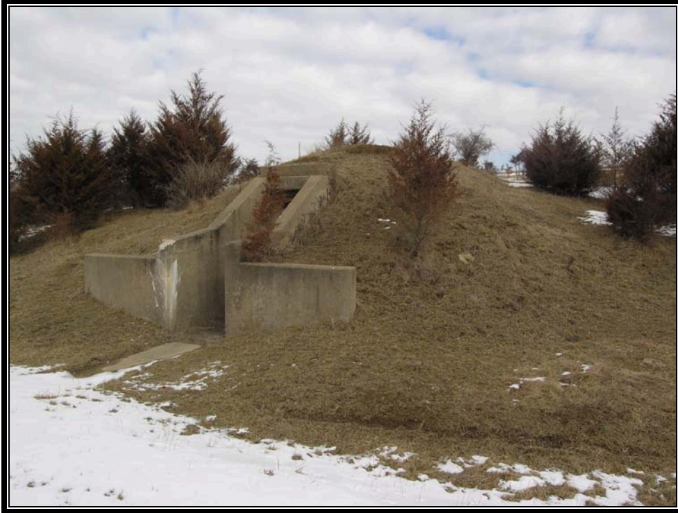
Plate 5.53 Typical frost-proof vault (Photo courtesy US Army, 2007)
