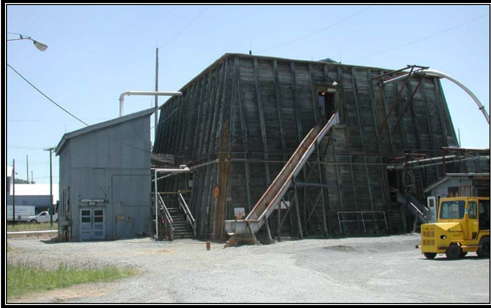
Plate 5.39 Typical solvent recovery building surrounded by Repauno barricade (Photo courtesy US Army)
