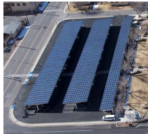
Figure 10. Carport-mounted Solar PV Panels at White Sands Missile Range, New Mexico
