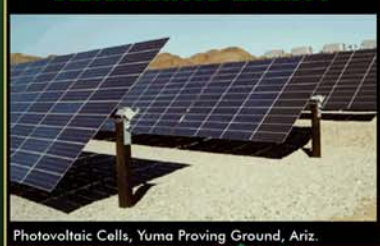
Photovoltaic Cells, Yuma Proving Ground, Ariz.
